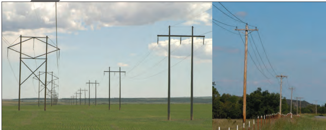
FIGURE 1.3: Transmission lines (left) and distribution lines (right).
